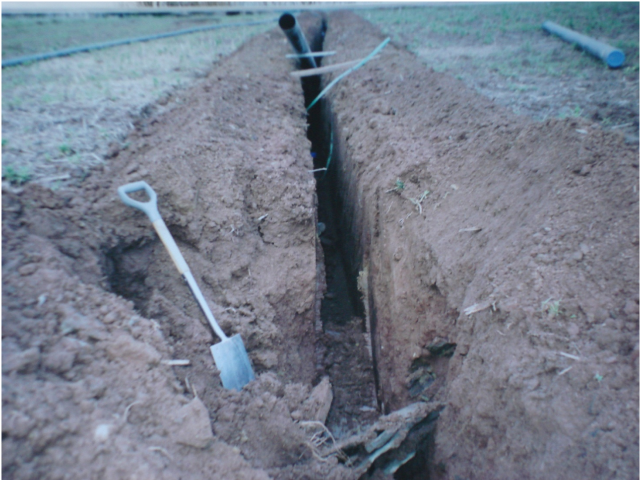
Figure 12: Extensive works to install irrigation pipes are agricultural operations and require no permission, but were argued to indicate the intended permanency of the tunnels they supply.
